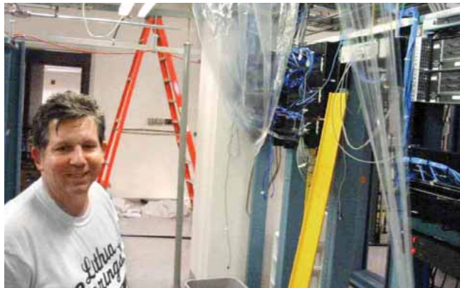
Technician Louie White protected T-Mobile gear from Katrina's wrath.
